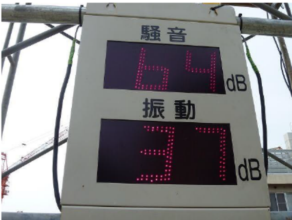
Figure 2: Sound level monitoring system for construction site in Japan.
